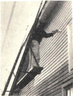
Always start painting a house on the north side. Work around so that the sun remains ahead.
